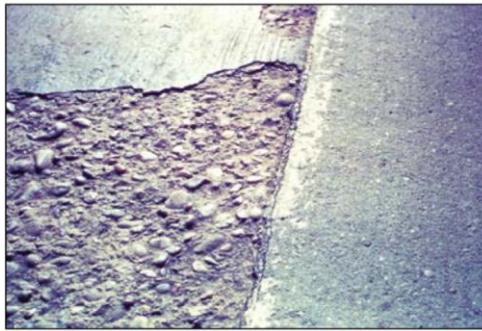
Gambar 9.15. Scaling pada perkerasan kaku (Sumber : U.S. Department of Transportation, 2014)
