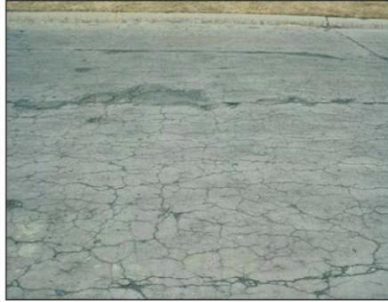
Gambar 9.14. Map cracking pada perkerasan kaku (Sumber : U.S. Department of Transportation, 2014)
