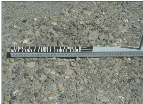
Gambar 9.9. Ravelling pada perkerasan lentur (Sumber : U.S. Department of Transportation, 2014)
